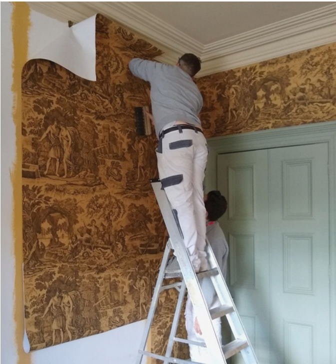
Fig.12 Watts & Co. Odyssey wallpaper, the design inspired by a French 18th century mythological toile fabric design, being installed in 2021 by Hesp & Jones
